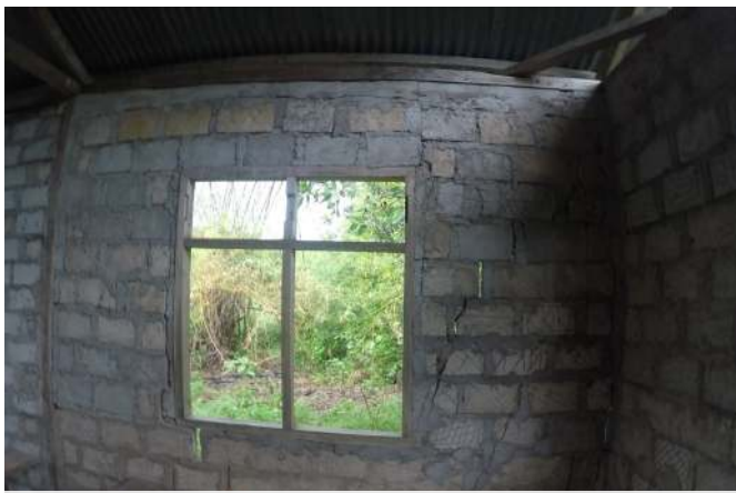
WatuPatah church cyclone damage
