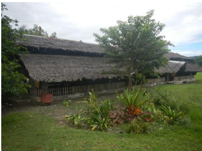
Current Living Water Christian School roof which is to be replaced with tin DV in the coming year
