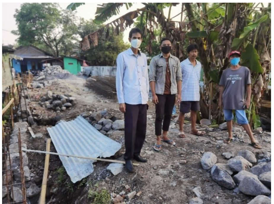
Rev Yanto, Ev Endrow & 2 congregation members inspecting new church foundations at Solo
